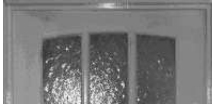
Figure 9: An unnecessary arch in a door(Flat lodgings)
