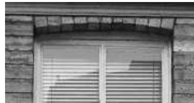
Figure 2: No matter how slight, there is an arch(ultimate window frame)
